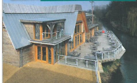
Pamela Jordan 'topping out' the Heritage Centre with an evergreen tree to mark the frame's completion
